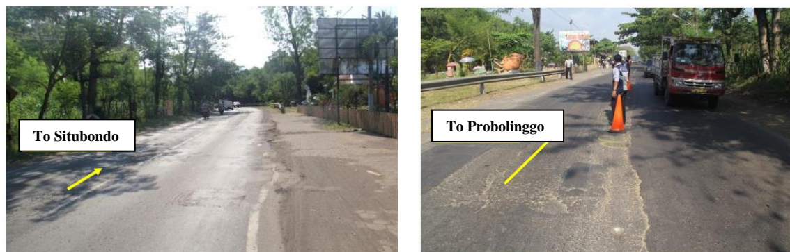
Figure 3. The condition of the pavement at the location of the incident
