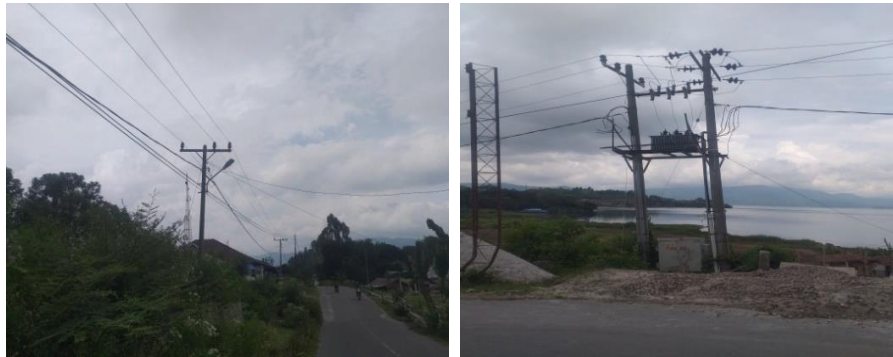
Figure 7. Electricity Network Condition in Tuktuk Siadong Village
