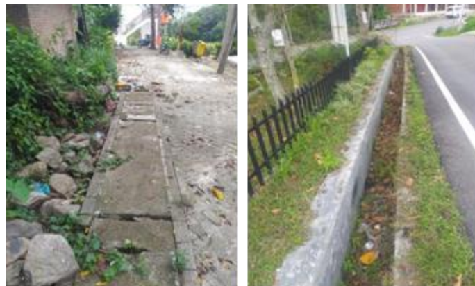
Figure 6. Condition of Drainage Network in Tuktuk Siadong Village
